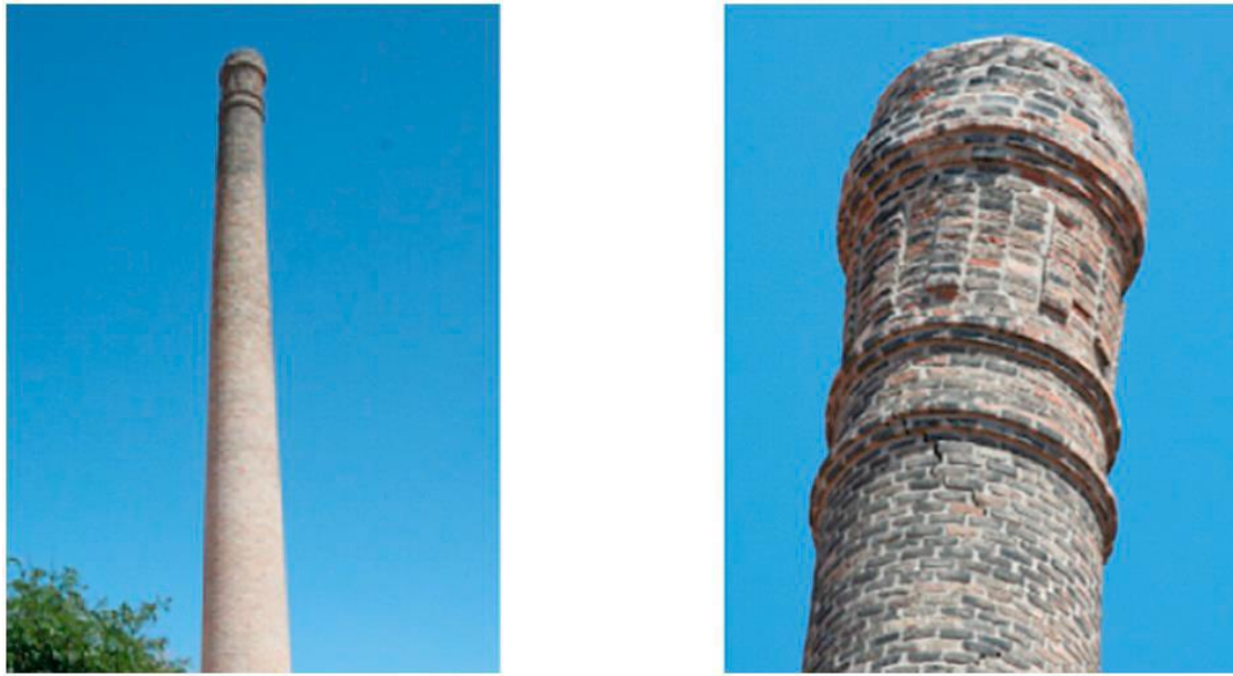
Figure 1: Failure of Chimney
