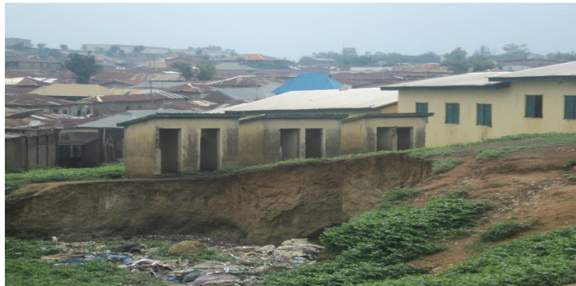
Plate 2 Public building damage due to effect waste disposal. Source: Author's fieldwork
