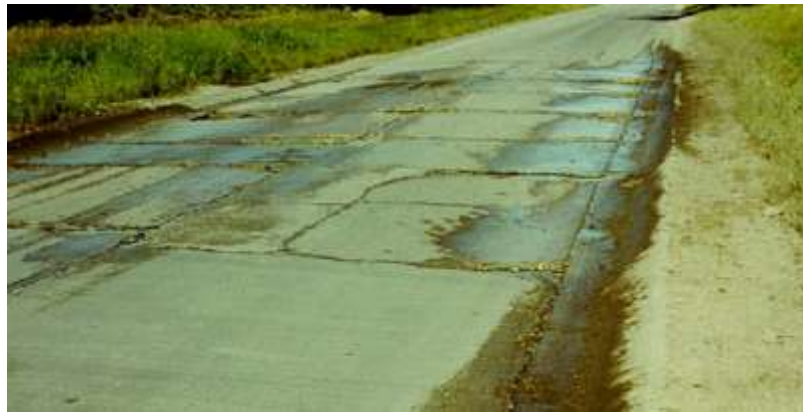
Fig.2 Mud pumping through joints/cracks in rigid pavements
