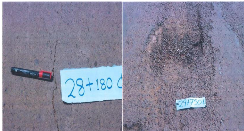
Plate 1.3: Crack in the surface that reflects light in a longitudinal direction Plate 1.4: Rumlblings about the surface and the potholes
