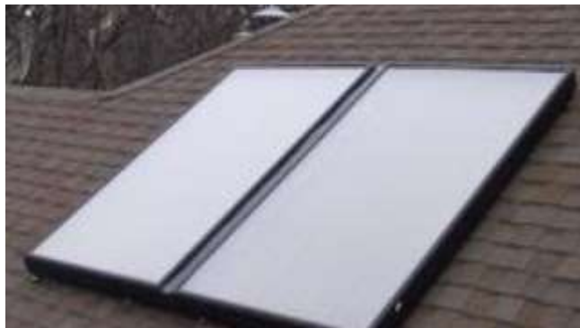
Figure 15. PV Solar panel
