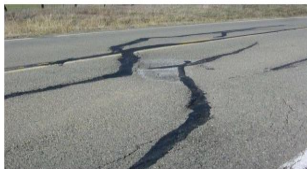
Fig. 1. Failure of highway constructed on B.C soil
