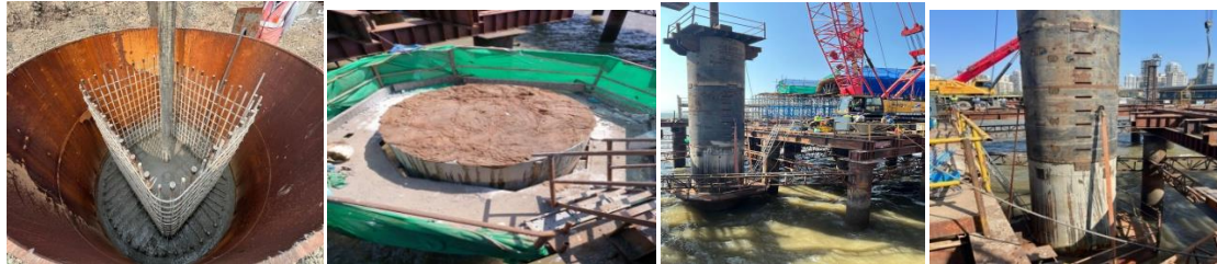
Fig Pile head concrete pou Prepared pile top for PDA. PDA test setup (offshore)fig PDA Sensors fixed at the platform level.
