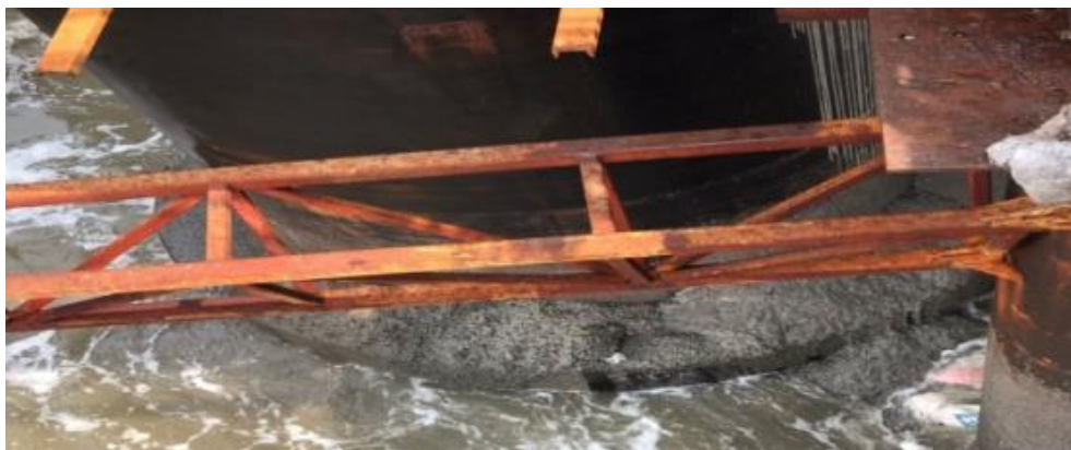
Fig Plug concrete between outer & inner liner to counter the wave impact on liner.
